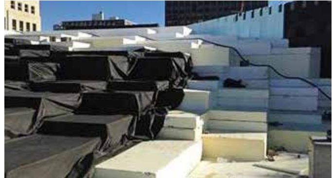
Figure 9. Geofoam blocks in use at the Alberta Legislature parkade in Edmonton, Alberta. Photo: EPS Molders Inc
